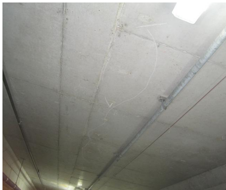
1련 Sta.0+52m 중균열(cw=0.2mm, L=4.0m)
