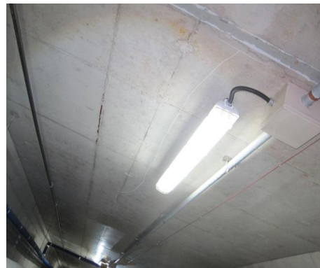
1련 Sta.0+87m 중균열(cw=0.1mm, L=4.0m)
